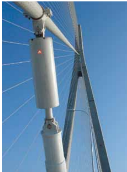
MAURER cable dampers, Sutong Bridge, China
