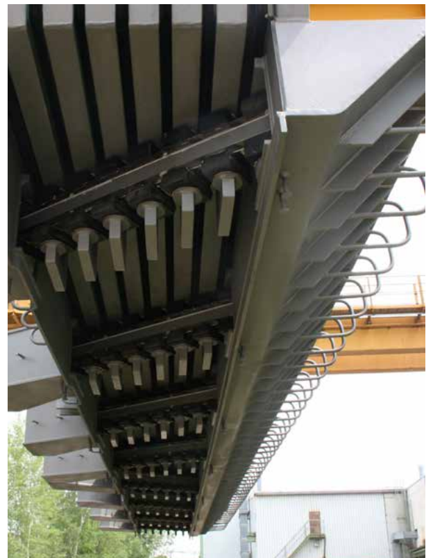
Type I Fuse Box System
