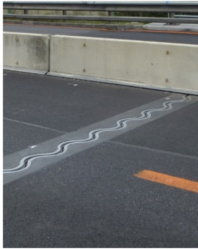
Motorway A21 Heiligenkreuz: Expansion joint XW1 with Betoflex® header
