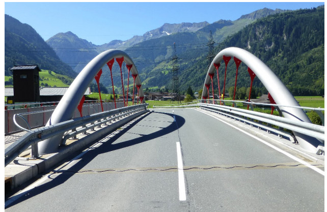
L264, Salzach Bridge Uttendorf, Austria: Expansion joints D1-B and XW1 with Betoflex® header
