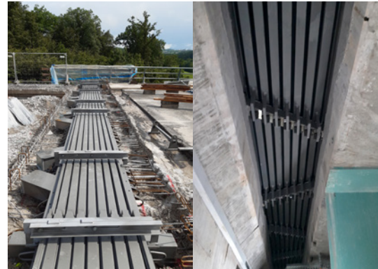
Left: The new MSM® Swivel Joist Expansion Joint during installation. It has a service life of over 100 years. Right: View from below of the new MSM® Swivel Joist Expansion Joint with the support bars arranged at an angle.
