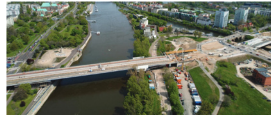
The Neue Strombrücke over the Elbe in Magdeburg during its rehabilitation in 2023. On the right, the second of a total of three bridges of the bridge structure.
