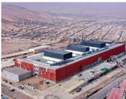
The clinic centre in Alto Hospicio in May 2021. The building structure is in place – entirely seismically isolated.
